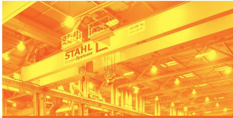
Five heavy duty cranes in engine production
